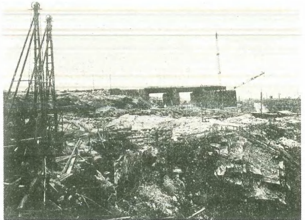
61. The Dniprel'stan (Dnieper Hydroelectric Station) was constructed in 1927-1932 under the on-site guidance of American engineers. The completion of this, one of the most ambitious Soviet projects of the first Five Year Plan, was made possible in part by the use of slave labor.
